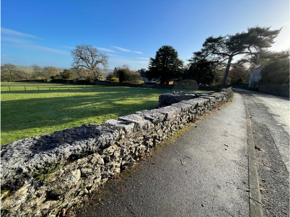
Figure 57: Limestone wall with flat coping, Yealand Road in front of Peterhill House and Laurel Bank
