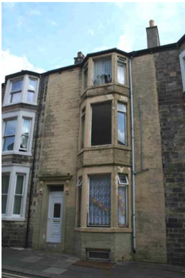
Inappropriate windows and door
