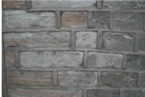
An example of bad pointing
