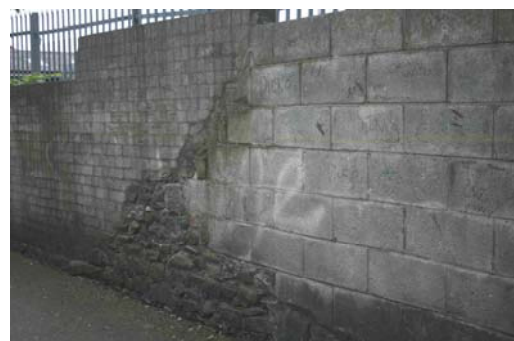
Inappropriate repairs on Church Walk
