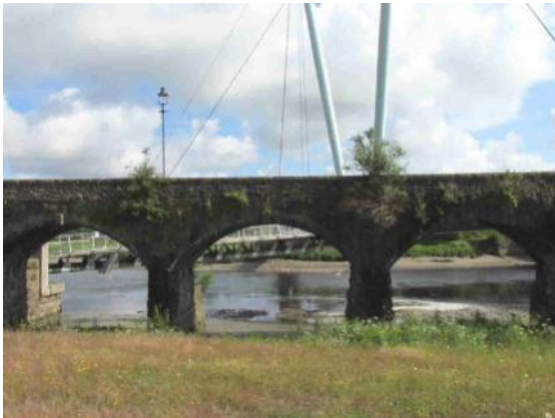
Vegetation growth on disused railway bridge
