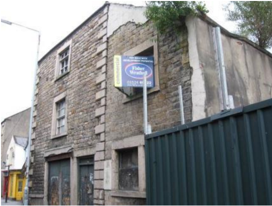
Neglected buildings on North Road
