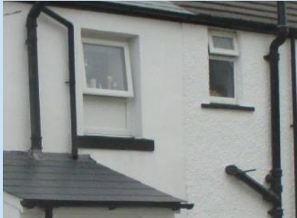
Fig. 29 Inappropriate top hung uPVC windows have a negative impact on the area.
