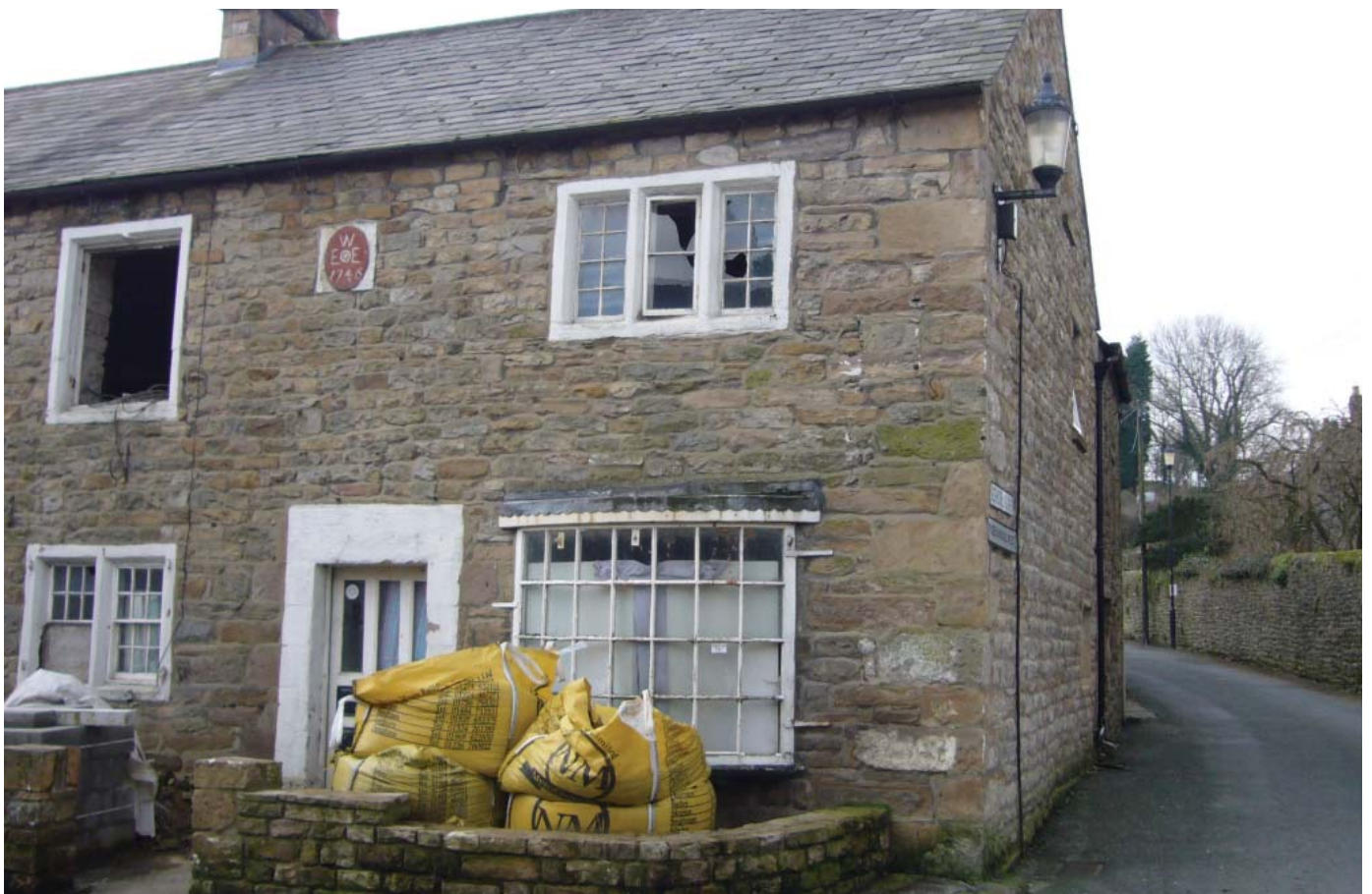
An inappropriate bay window and poor condition detract from this cottage of 1746
