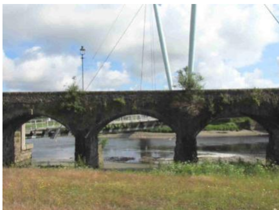
Vegetation growth on disused railway bridge
