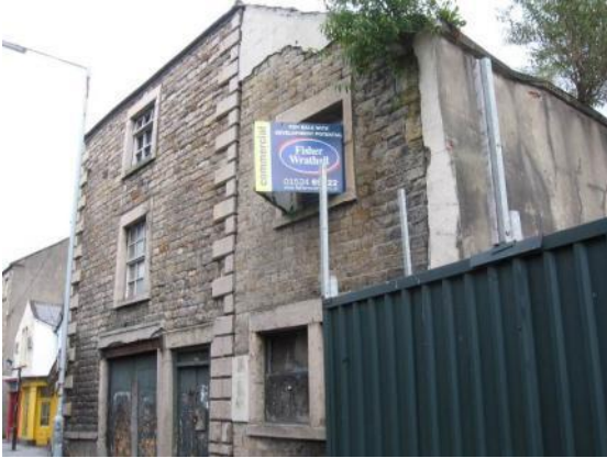
Neglected buildings on North Road
