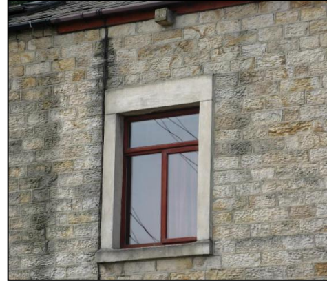
Inappropriate window styles
