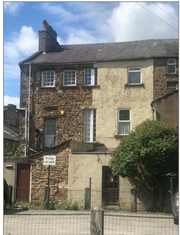
Rear of no.s 37 and 39 North Road. Central bay, including stair window, divided.
