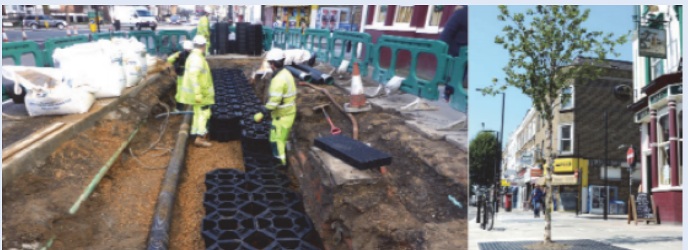
Recycled plastic flexible soil support systems connecting SuDs tree pits from one side of the road to another (left), and the SuDs tree pit when completed (right). Photo by GreenBlue Urban.
